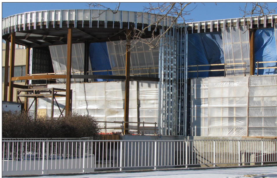
IN PROGRESS: Work continues on the new College of Pharmacy building on Health Science Campus. The $25 million facility is slated to open this summer.
