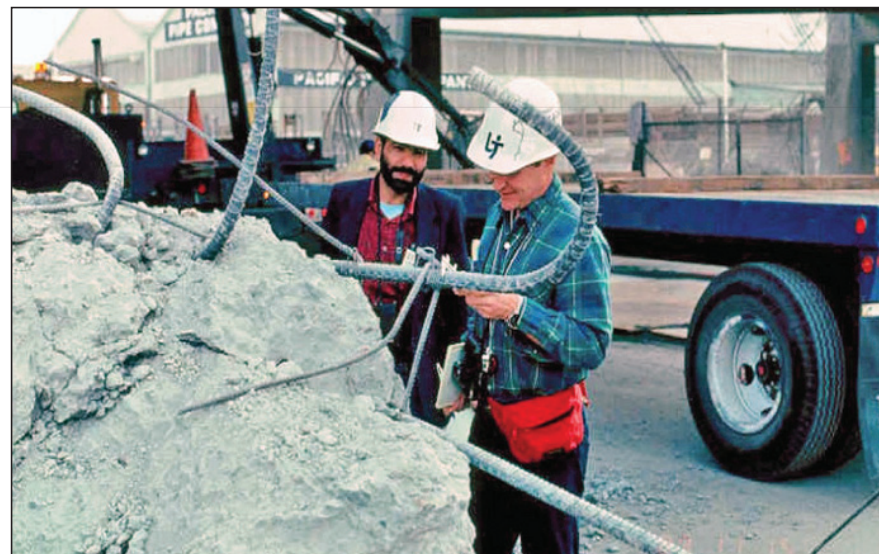
DAMAGE ASSESSMENT: Dr. Mark Pickett, right, and then UT doctoral student Dr. Omar Abu-Yasein examined a failed column from the I-880 bridge that collapsed during the 1989 San Francisco earthquake.
