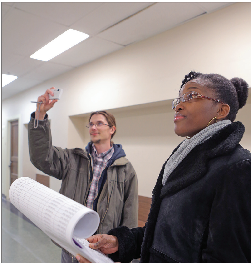
LIGHTEN UP: Sandrine Mubenga, UT electrical engineering manager, and her team of staff and students are moving to University Hall to outfit some 2,300 occupancy sensors, which will turn lights on or off based on room use, and about 9,000 lighting fixtures. Support for this project came from Peak Lighting, Gross Electric, Laibe Electric, FirstEnergy Toledo and the state of Ohio.
